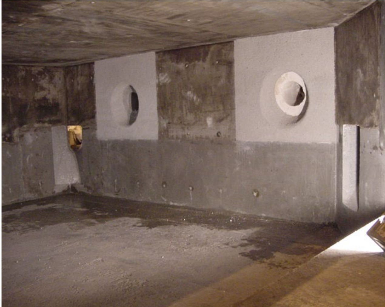
40T Holding Furnace - UK
